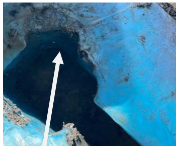
Deformation around the fixings
