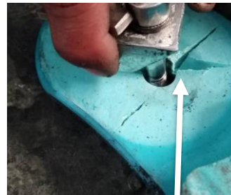
Cracks near the fixings
